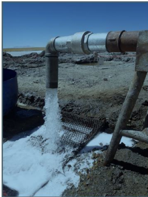
Figure 7.56 Pumping Well W18-05
