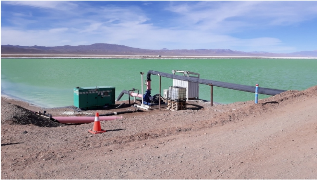
Figure 14.6 Evaporation Ponds – Transfer Pump Station
