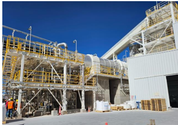
Figure B: Completed the first train of the KCI plant with commissioning underway.
